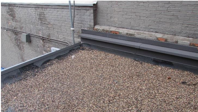
Lack Of Safety Rail on Leading Edge of Lower Roof
