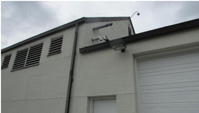
Ice Build Up During Winter Over Ped Door to Garage
