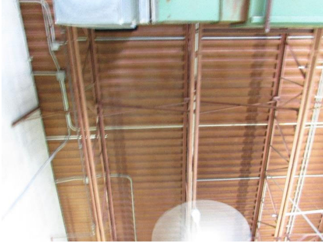
Rm 115 – Garage – Red Dust Falling from Ceiling
