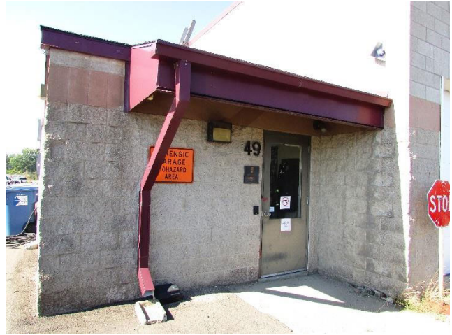
Ice Accumulation in Front of Door During Winter
