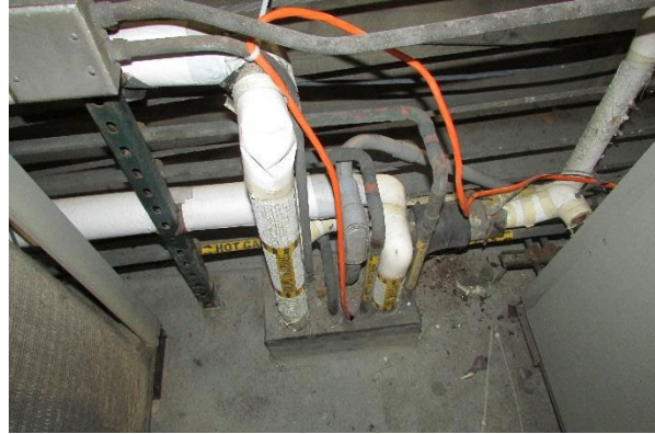
Electrical Installation for (Presum.) Cond Unit (Pic 2)
