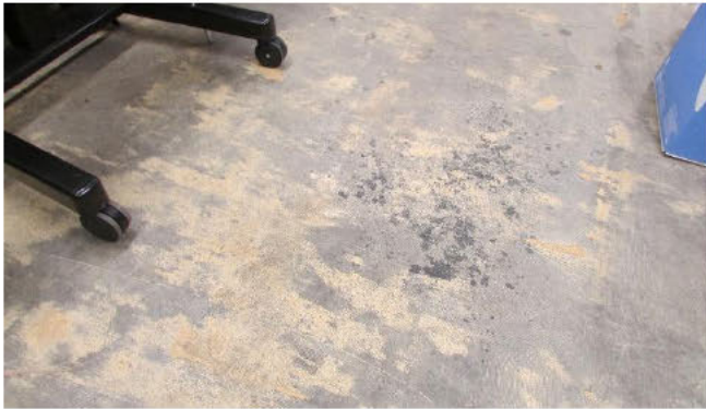
Rm 105 – Training Storage – Missing VCT
