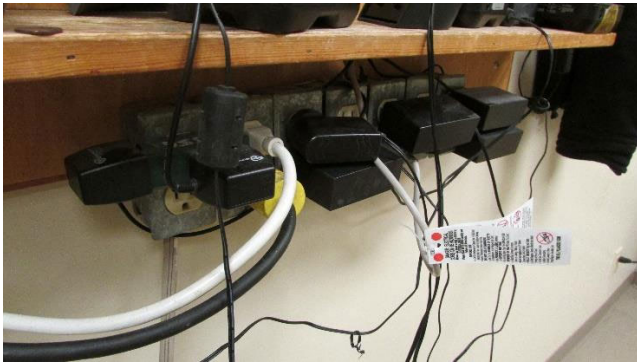
Overloaded Outlets in Men's Locker Room
