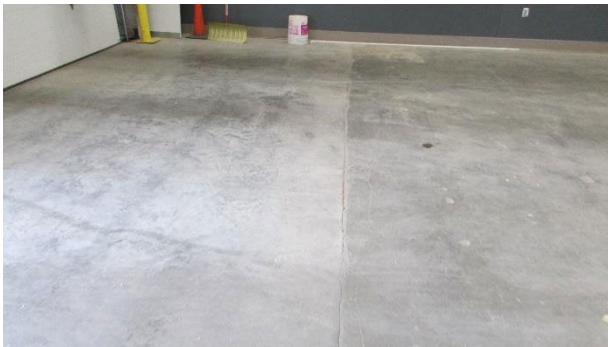
Garage Bay Drainage Sloping Inward
