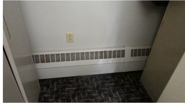
2 nd Floor Cubicles Against Fin Tube Radiation
