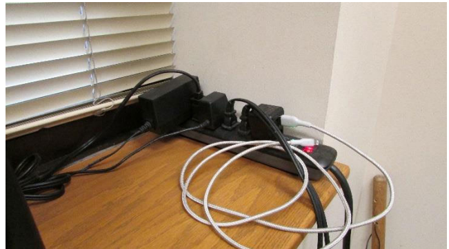
Extensive Use of Electrical Power Strips
