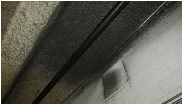
Garage: Black Residue (Presumably) From Exhaust
