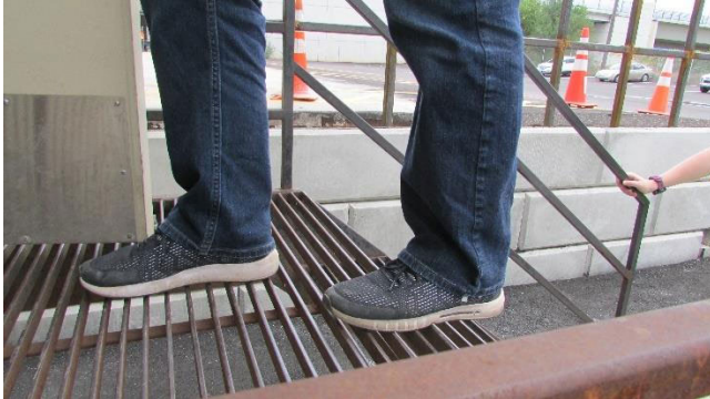
Rear Stairs Size Preventing Safe Opening of Door
