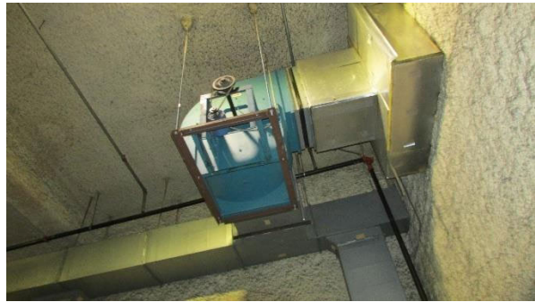
Garage: Existing Garage Exhaust Fan
