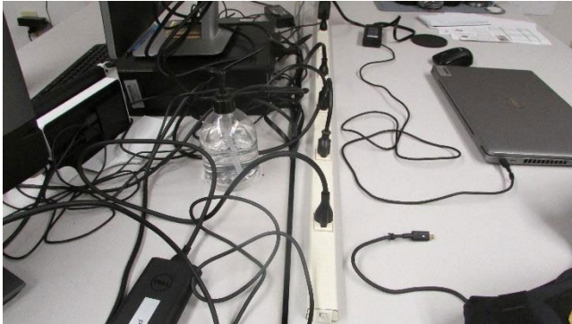
Extensive Need/Use of Power Strips
