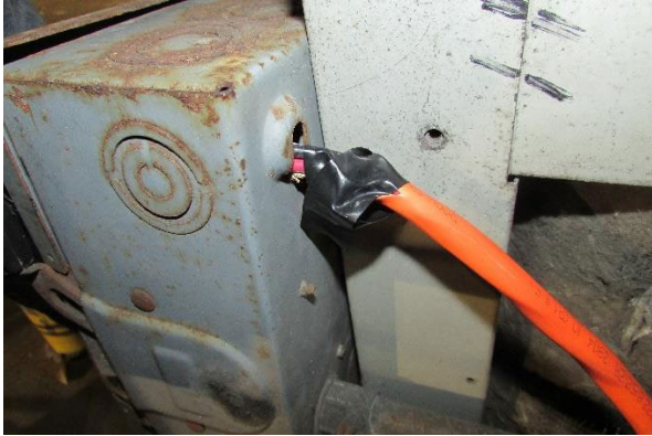
Electrical Installation for (Presum.) Cond Unit (Pic 1)
