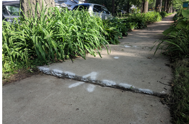
Figure 3-17: Vertical fault due to a heaved panel, likely from tree roots. This panel is marked for replacement through the city’s Defective and Hazardous Sidewalk Repair Program (SWK01).
