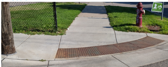
Figure 3-3: Fan Ramps or Depressed Corner Ramps provide one ramp to cross the street in either direction
