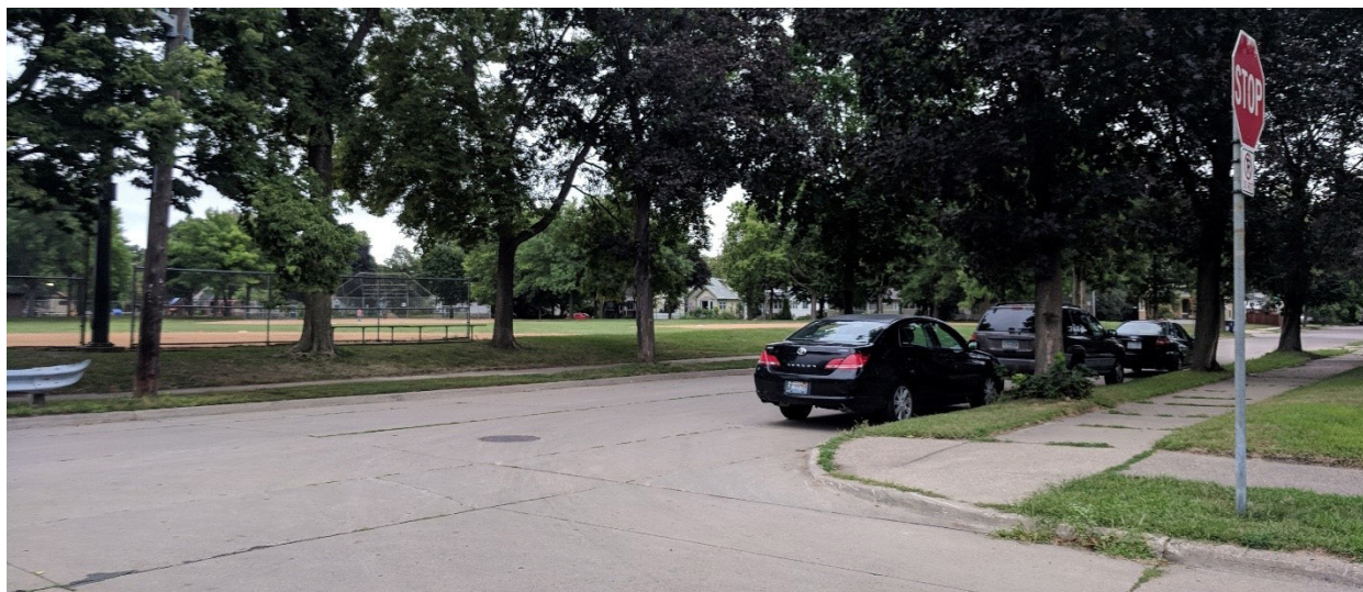
Figure 2-6: Pedestrian ramp missing in distance between far sidewalk and existing crossing
