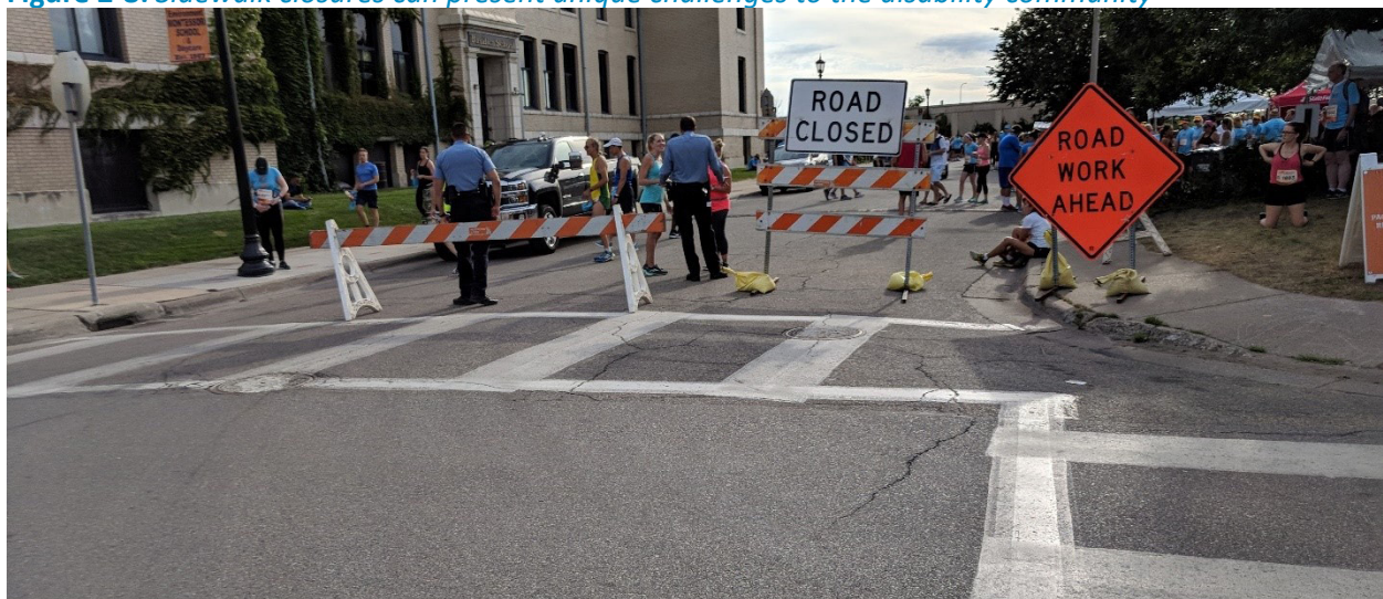
Figure 2-8: Sidewalk closures can present unique challenges to the disability community
