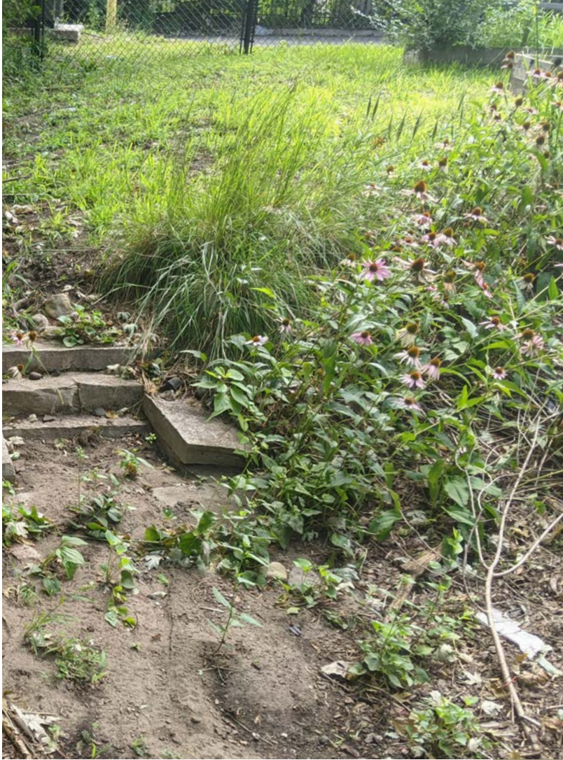
Pond inlet sedimentation needs maintenance. Photo Credit: Metro Blooms Design + Build
