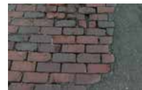
Logan Park pavers with asphalt over the utility trenches
