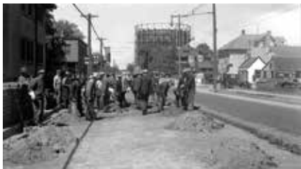
Installing brick pavers, looking west on Broadway toward Central Avenue, ca. 1930s. Gasometer at right background.
