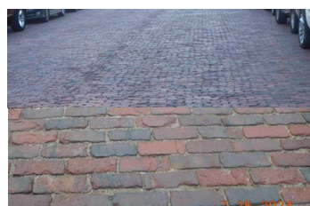
North Loop- 4 years later bricks are breaking up/ failing
