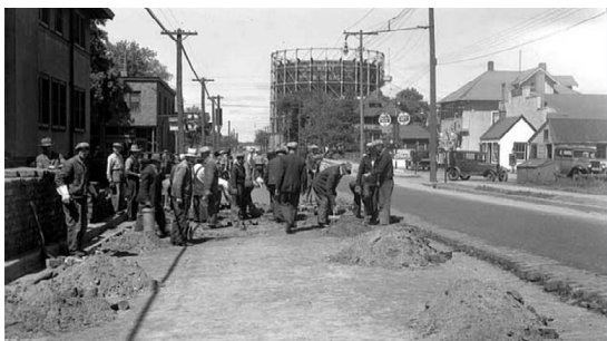
Installing brick pavers, looking west on Broadway toward Central Avenue, ca. 1930s. Gasometer at right background.
