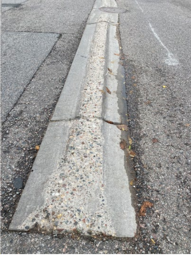
Figure 6: Damage on the raised hardened centerline at Fremont Ave N & 42nd Ave N
