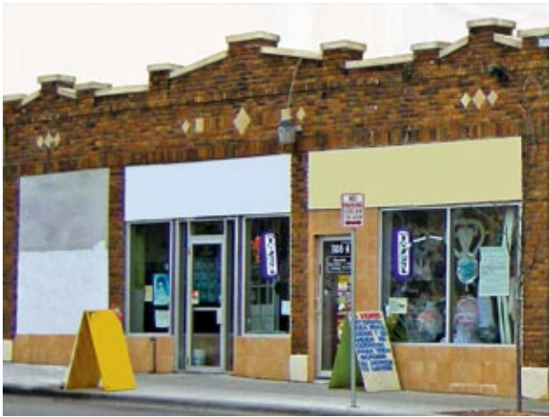
BEFORE Covering windows and skirtboard panels with boards or other materials is discouraged.
