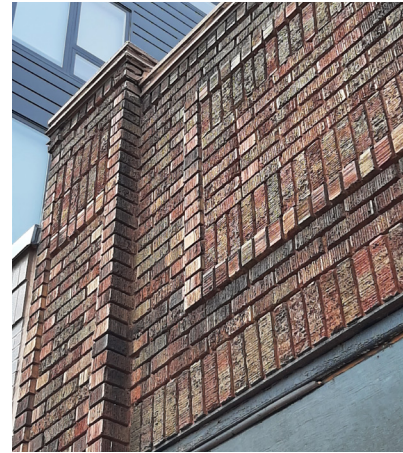
Masonry is a common wall material throughout the district. Notice the different bond patterns. This wall has stretcher bond, soldier courses, header courses, and stacked bond.
