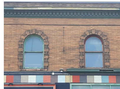
Note the arched window openings on the second story of 325-331 14th Ave SE. They reflect the building's Renaissance Revival architectural style.
