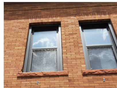
These replacement metal windows at 1401-1411 4th St SE are set within the historic openings. The jack arches above and sills below are original.
